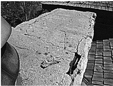
Damaged Chimney Cap
