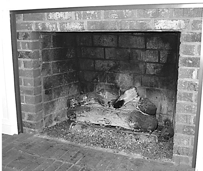
Masonry Woodburning Fireplace
