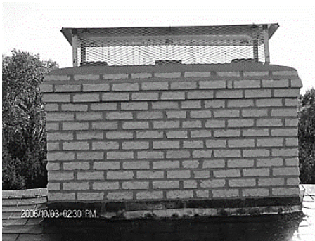
Metal Cap on Clay Liner Chimney Top
